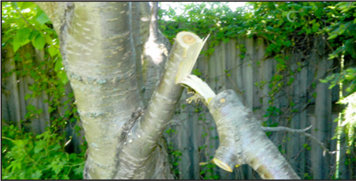
This rip cut is caused by sawing from the top of the branch.
