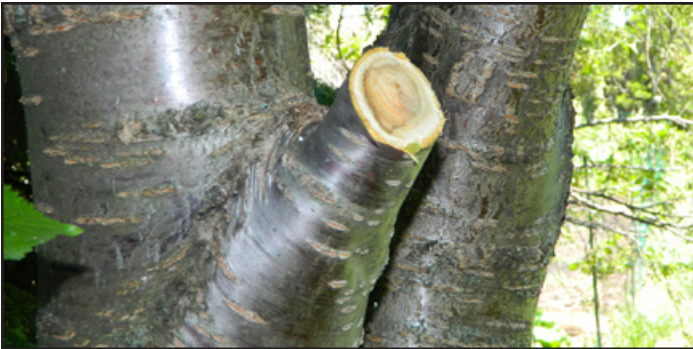
A stub cut leaves a small portion of the branch, which promotes decay.
